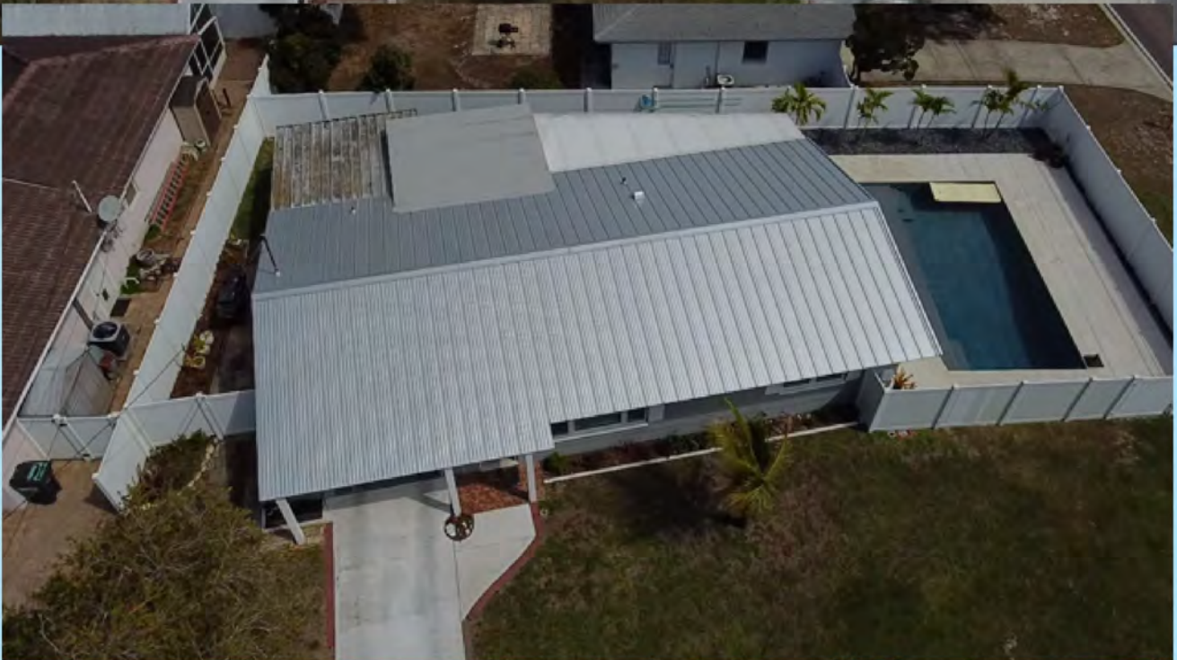
Standing Seam Metal + Modified Bitumen, Tapered
