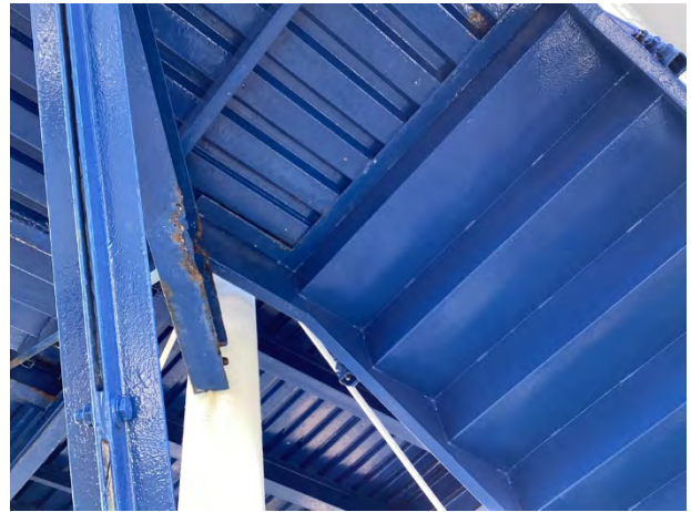
Rusted staircase structure
